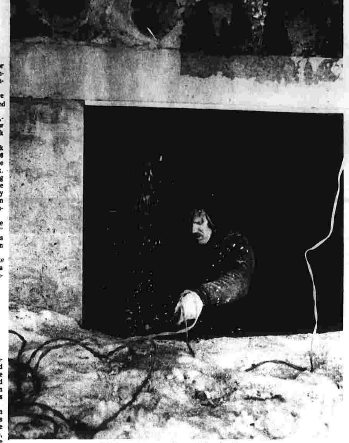
Chips ice to install window Jim Bousfield of Manchester, an employee of Tim Connelly, general contractor, chips ice to install a window in the new addition to the Church of Christ. (Herald photo by Dunn)
