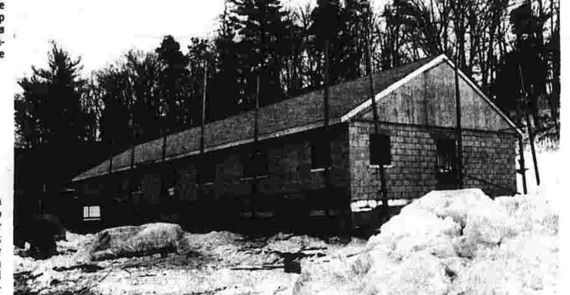
Addition nears completion This addition to the Church of Christ, located at Vernon and Lydall streets, is nearing completion. The construction is being done by Tim Connelly, a Manchester general contractor. (Herald photo by Dunn)
